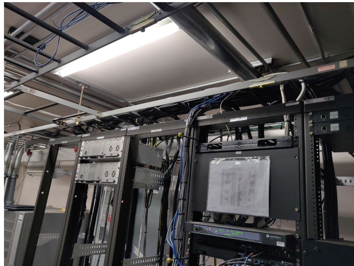
Network Room inside Ravinia Tower (Non-MARTA)
