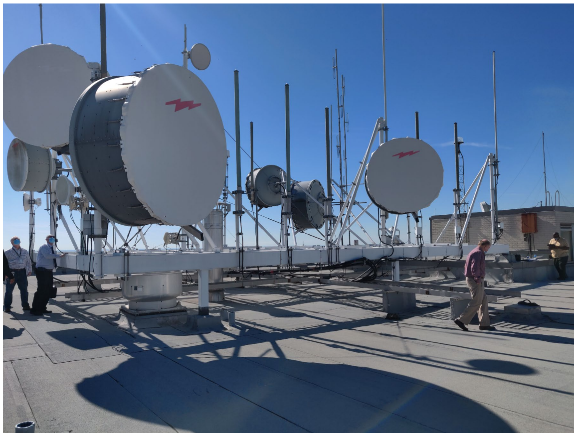
Existing Microwaves (Non-MARTA) on Ravinia Tower
